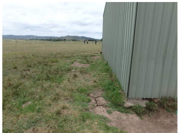
Plate 6. Localised erosion causing runoff of silty topsoil under shed eaves, view north.
